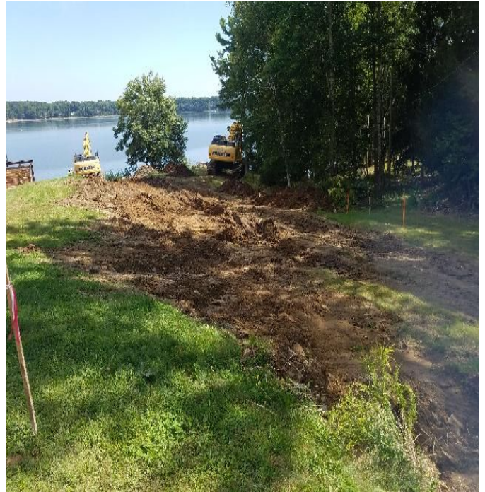
Fig 6: Blu Rock beginning trench excavation on the west side of Little Bay. Viewing west. (9-3-19).
