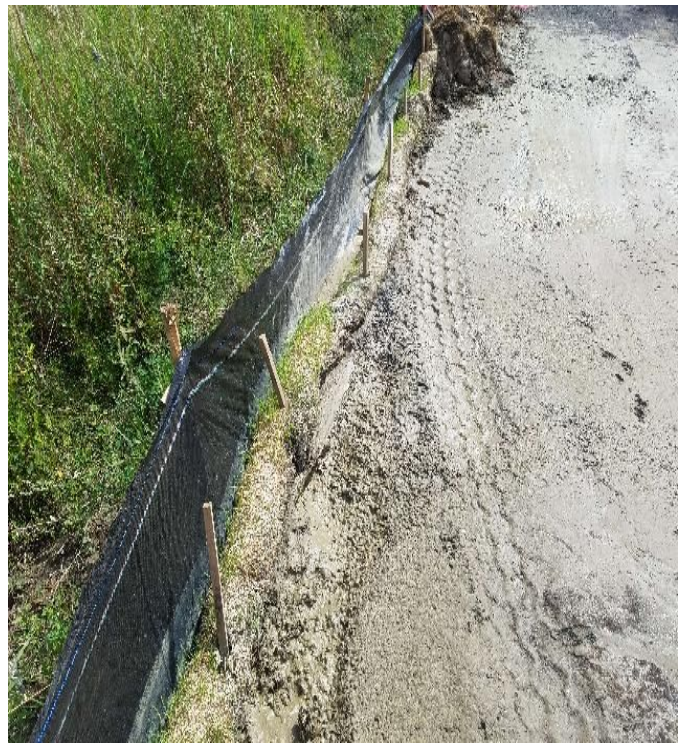
Fig 18: Erosion controls installed at Waterworks Rd parking lot needs to be repaired.
