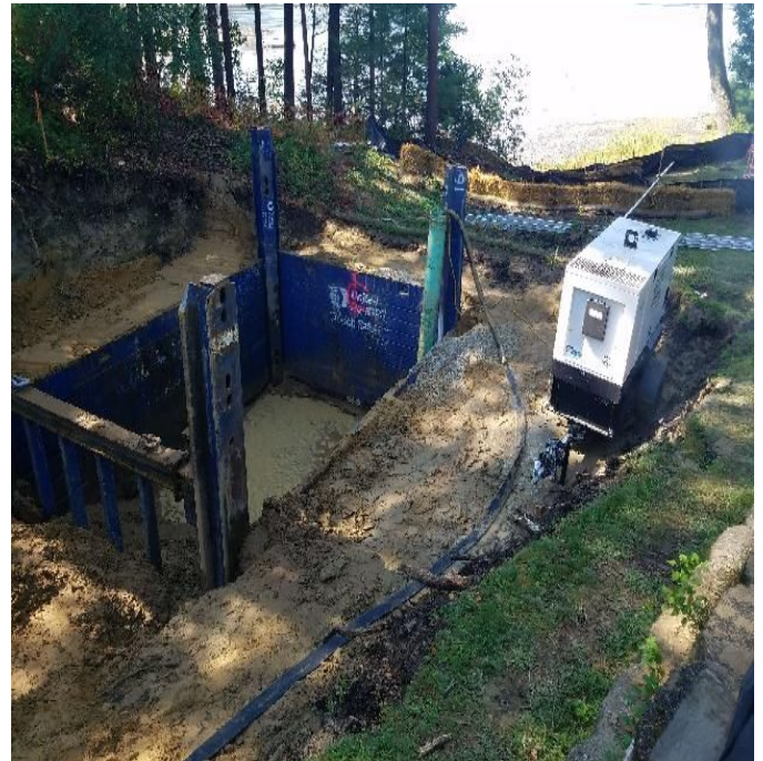
Fig 10: Pumping water out of manhole and into treatment tank at Gundalow Landing. Viewing south. (9-3-19).
